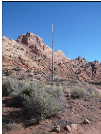
Travelers' Information Station Antenna at Entrance to Arches National Park, Utah
